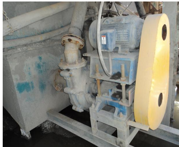
Goulds 125 XHD pump installed on oxides/sulfides slurry mill discharge at a silver mine in Northern Mexico. The customer built the adaptor base under the pump in order to align the pump flange with the suction piping.
